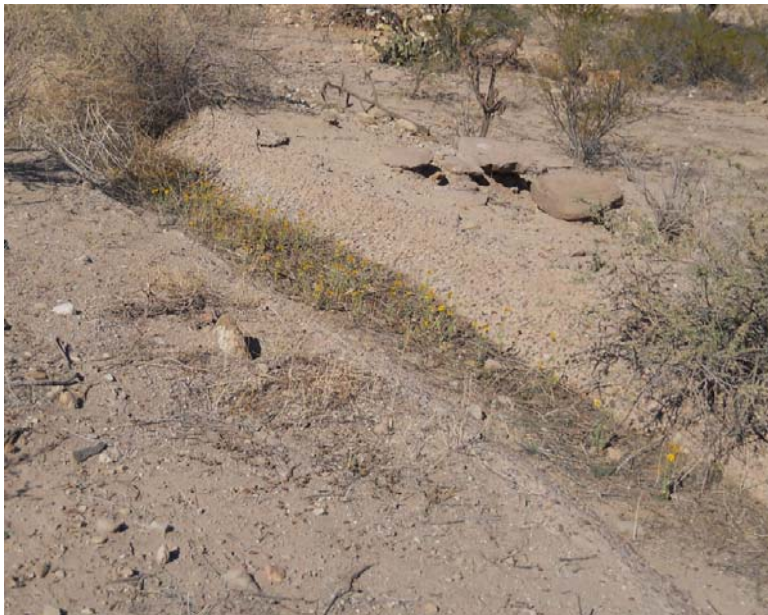
TRANQ2 – A closeup of the historically reworked coarse aggregate canal lining that resembles similar rework on the Marijilda Canal. The view is to the north at 32.76485 -109.72952 .
