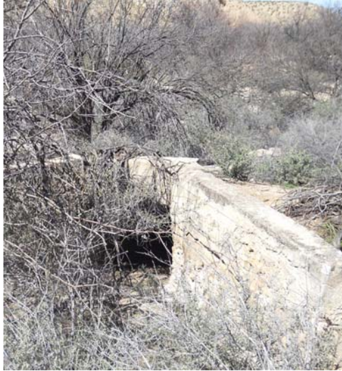
CLLUFFNW1 – One of several Y-Weir concrete structures from the second historical rebuild of the Cluff NW canals. This one was apparently part of a wash crossing inverted siphon. Viewed northwest from N 32.82647 W 109.84590 .
